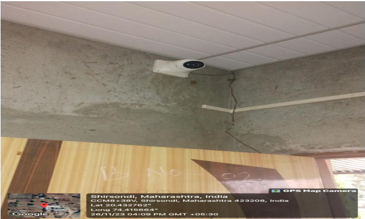
CCTV Camera - Class Rooms
